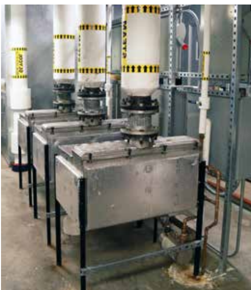
Vaporstream humidifiers Three Vaporstream humidifiers providing humidity in a performing arts center.
